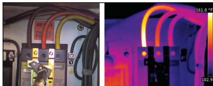
The above image is an Infrared Scan showing a loose electrical connection
